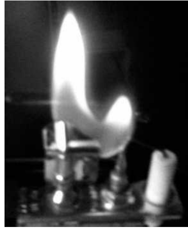
Right yellow flame incorrect aeration hole needs cleaning
